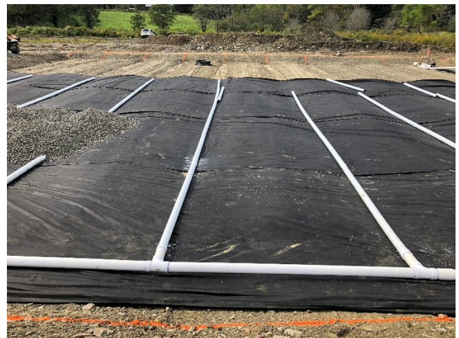
Geotextile placed over subgrade, under perforated pipes. Along bottom of photo is the solid PVC collection pipe, placed at -1.0% grade from left to right.
