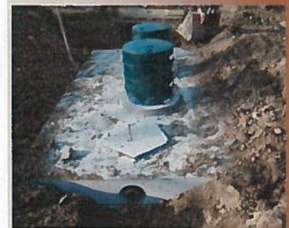
Buried holding tank for woodchip pad drainage water. Water is dosed from tank to adjacent vegetative treatment area.
