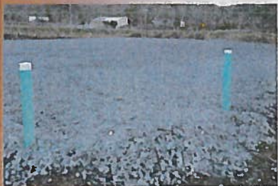
Drainage stone is placed over the perforated pipe. Accessible clean-outs are recommended to protect against clogging.
