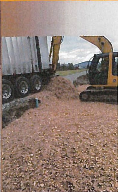
Woodchips being unloaded with a live-bed trailer, and spread with an excavator during construction.
